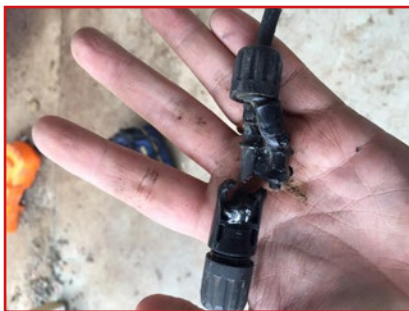
Fig. 2: Low Quality DC cable with burnt connectors
